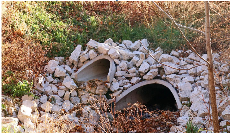
The large culvert that Karen and her friends were fond of exploring in winter has been replaced by two culverts.
